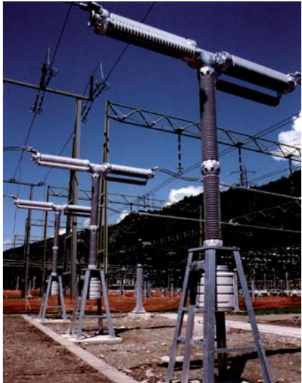
420kV life tank breaker
