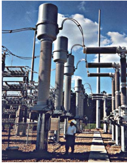
420kV instrument transformer
