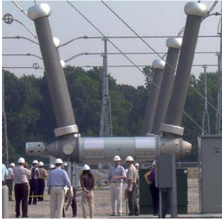
800kV dead tank breaker
