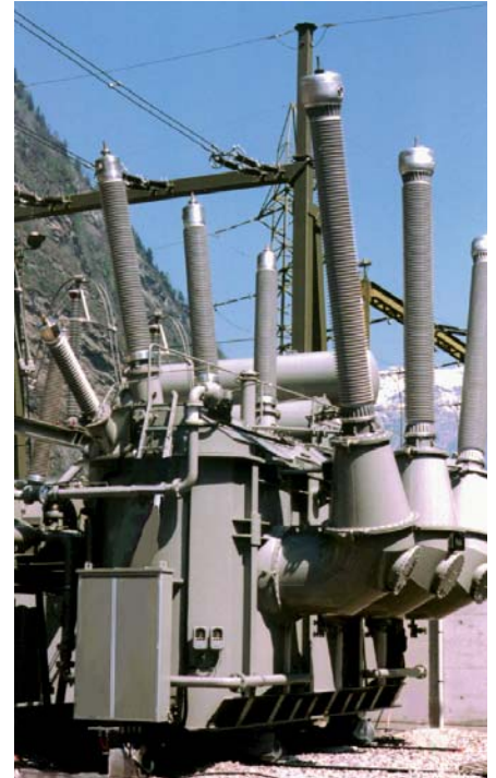
420kV power transformer
